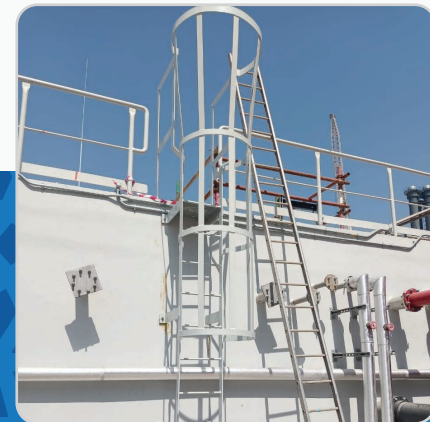
Cage Ladder & Handrails
